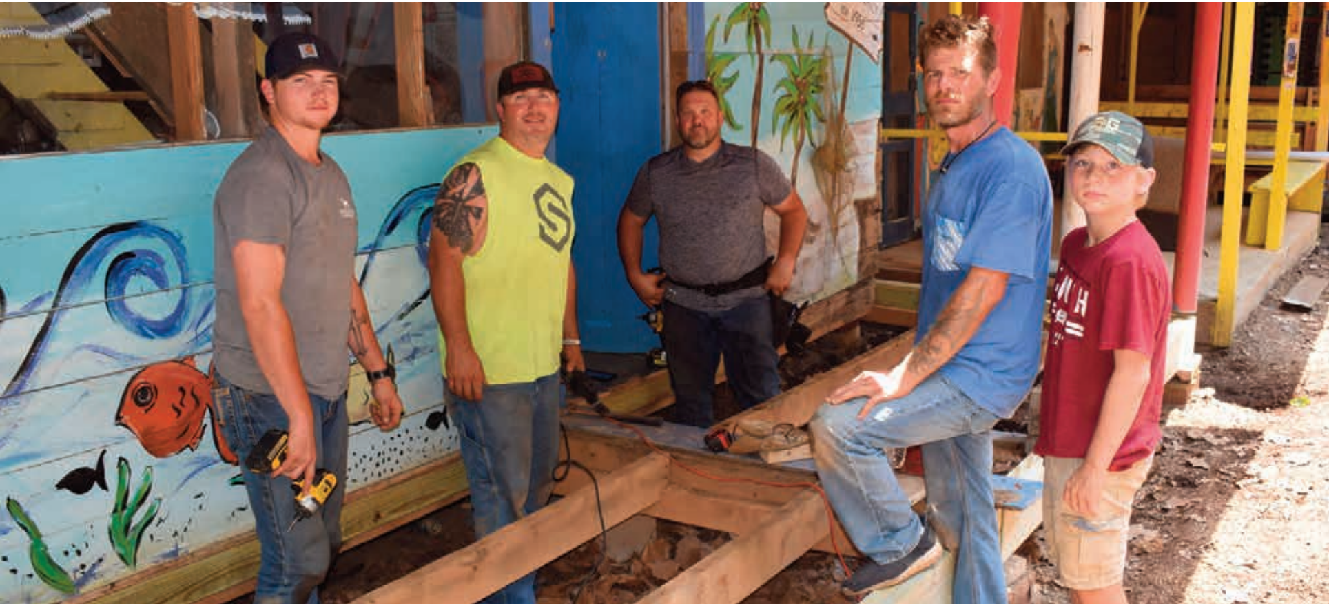
Jacob Hughes, Justin Pitts, Trent Rideout, Bubba Crapps and Zack Allen build a porch for a cabin.
