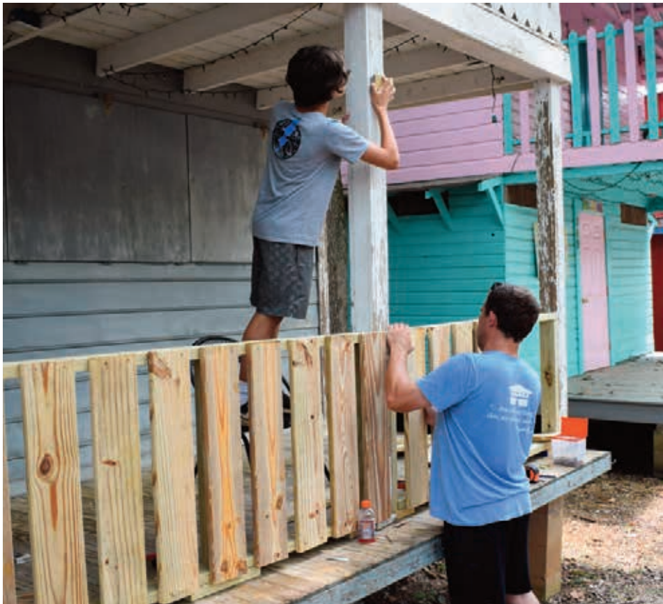
Cullen and Cory McCoy paint and repair their deck for this year's Fair.
