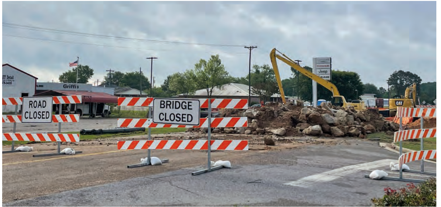
Motorists are told by officials to expect some traffic slowdowns on Highway 19 south due to bridge work.
