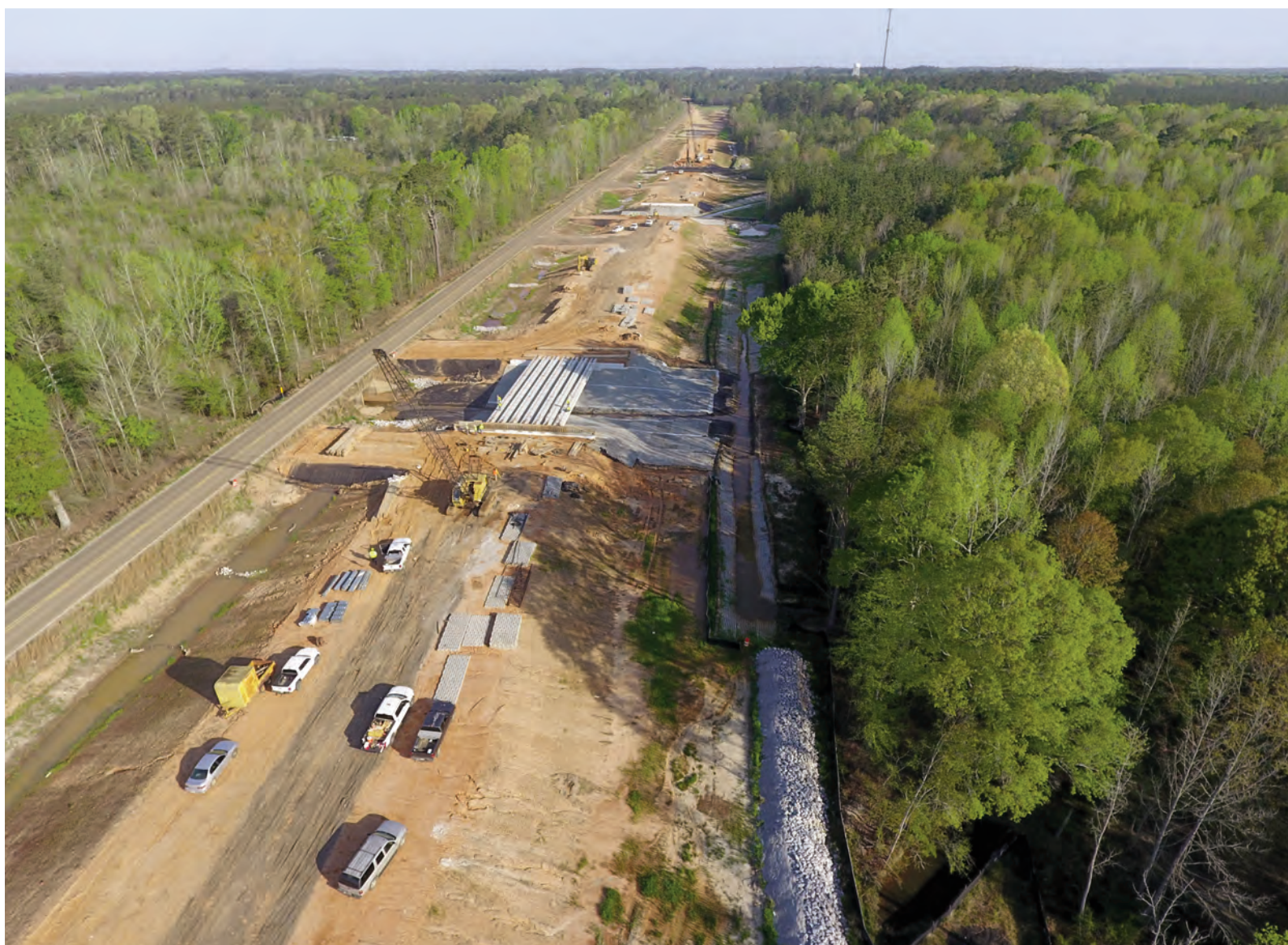
An $11.7 million two-lane bridge replacement at Tucker will be completed this fall. — Photo by Jonathan Addy
